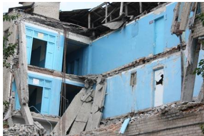
Fig.1.12. The collapse of the building's roof, floor and part of the walls of the façade in the building of the Lyceum in Kirovskoe town, Donetsk region, Ukraine
